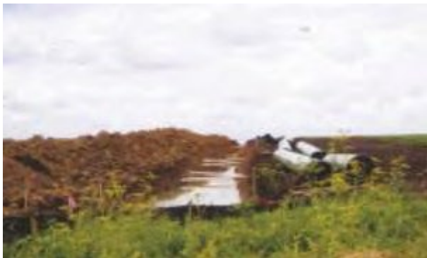
Photo 11: Impacted drain tiles that have been temporarily repaired allowing them to function until permanent repairs can be made
