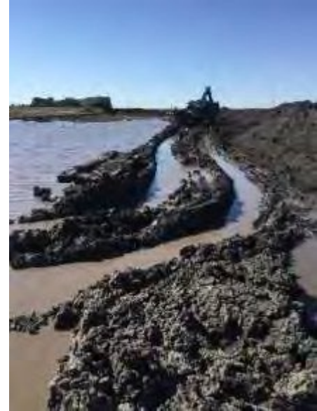
Photo 2: After topsoil has been removed, tracking through saturated subsoil may cause damage to drain tile
