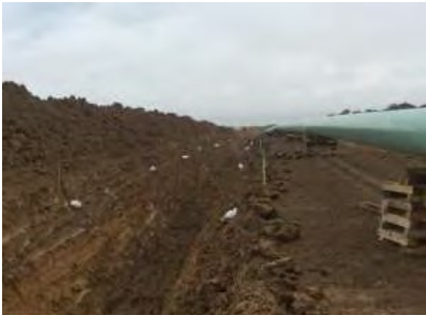
Photo 10: All impacted drain tiles are properly marked with stakes and screened with white filter bags
