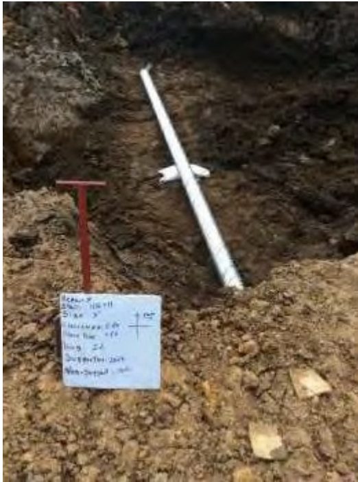
Photo 12: The permanent tile repair has been properly supported by sandbags and with a rigid pipe that spans across the ditch line
