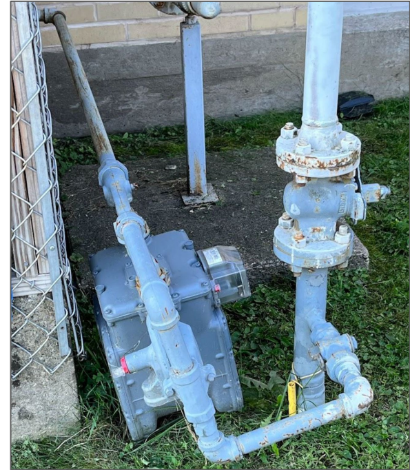
Example of stressed meter piping
