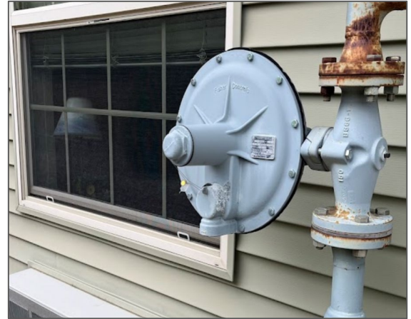
Example of vent near window
