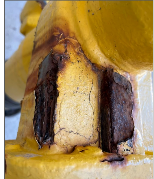
Metal Loss on Service Valve
