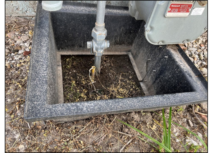
Example of buried crimp identified in 2024 inspection
