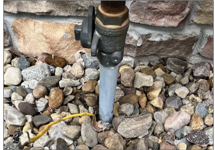
Example of buried anodeless riser crimp identified in 2024 inspection
