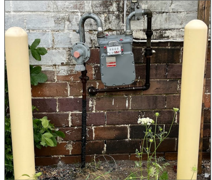
Example of stressed meter piping
