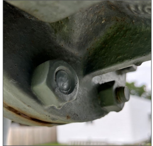
Example of short bolts identified in 2024 inspection
