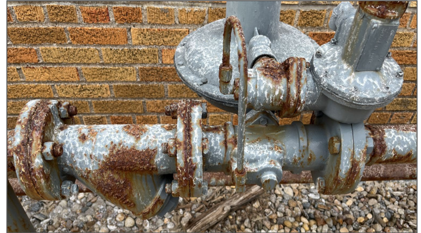
Example of atmospheric corrosion at meter set
